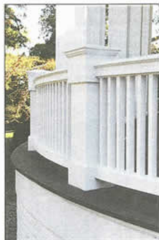
Georgoutsas also custom-milled balusters, posts and rails — all painstakingly done in his Bergenfield shop — to replicate the originals.
